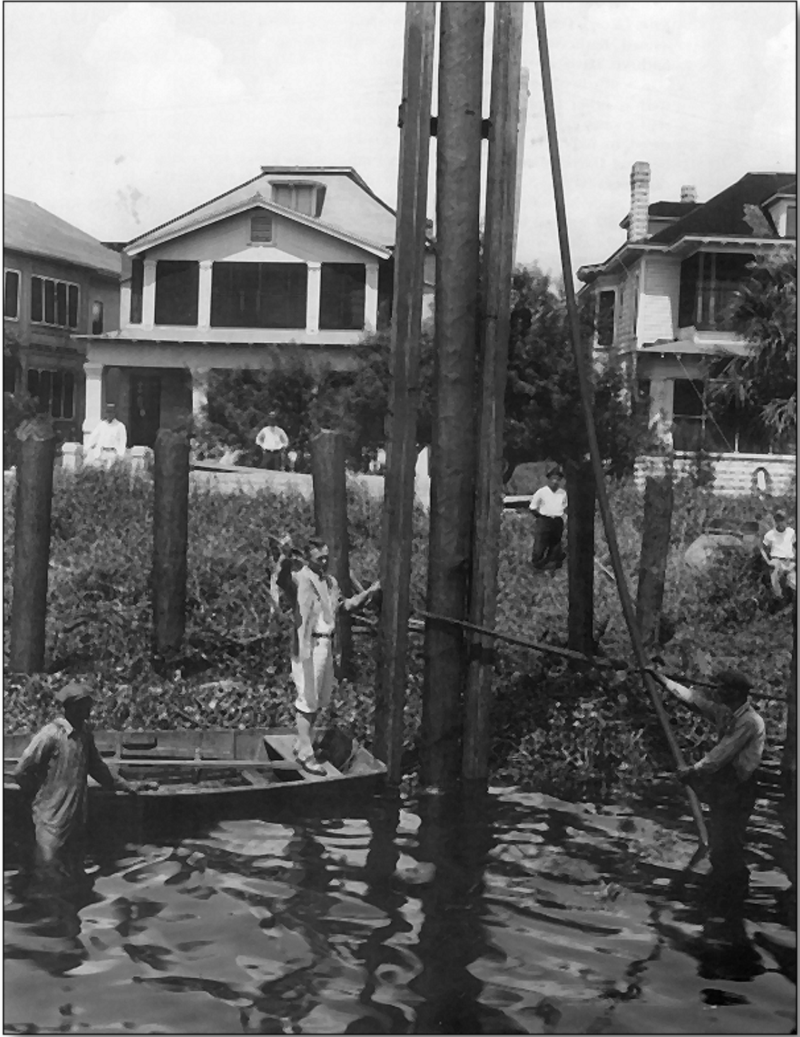
David Paul Davis is shown standing in a small skiff directing the placement of pilings for the first wooden bridge built to the islands. Homes along the Bayshore and curious bystanders can be seen behind Davis. This photograph and the one on the facing page appear to have been taken during the same Burgert shooting session.
